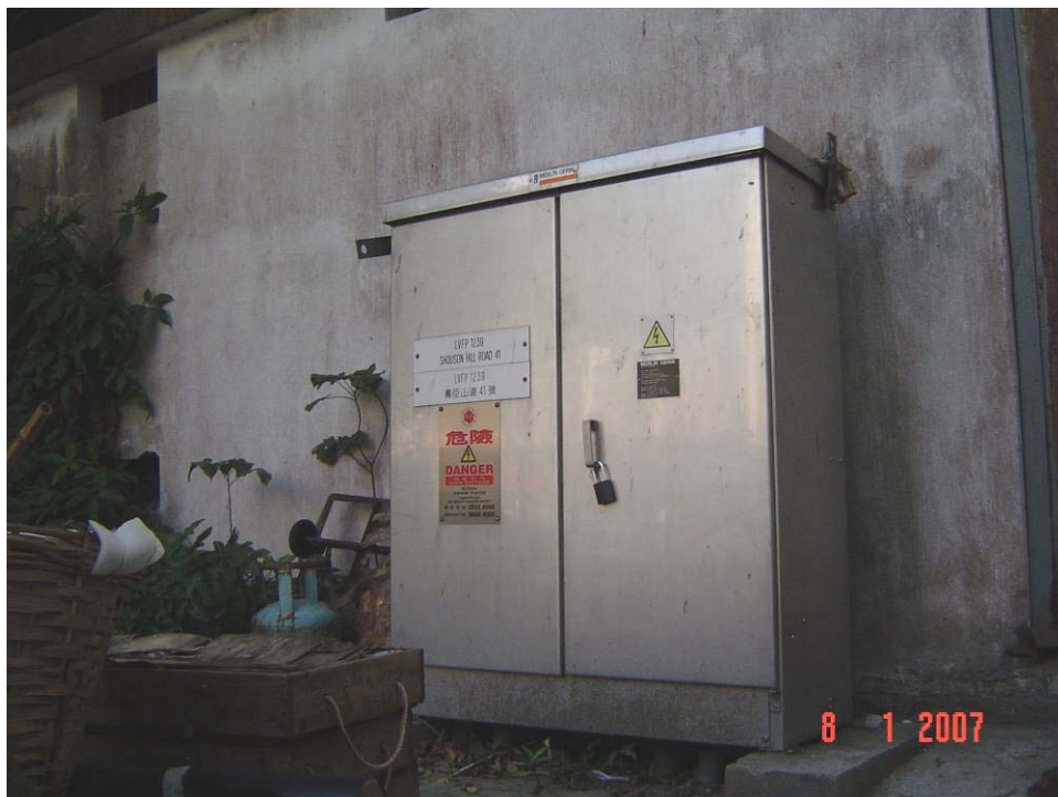
Photo 18 – LV Fuse Pillar
