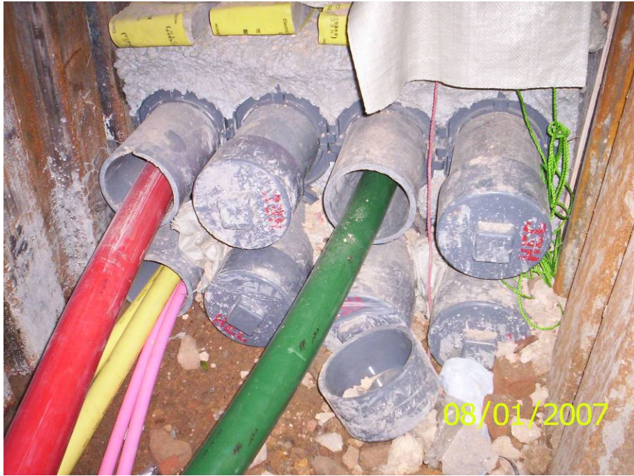
Photo 5 - 11kV, LV and Communication Cable Ducts
