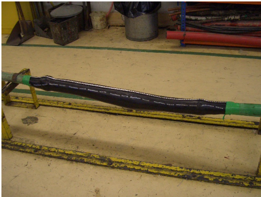
Photo 6 - LV Cable Joint
