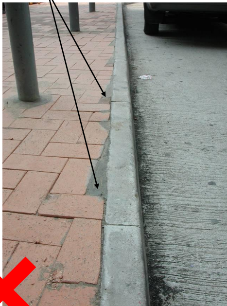
Unsightly concrete infill
