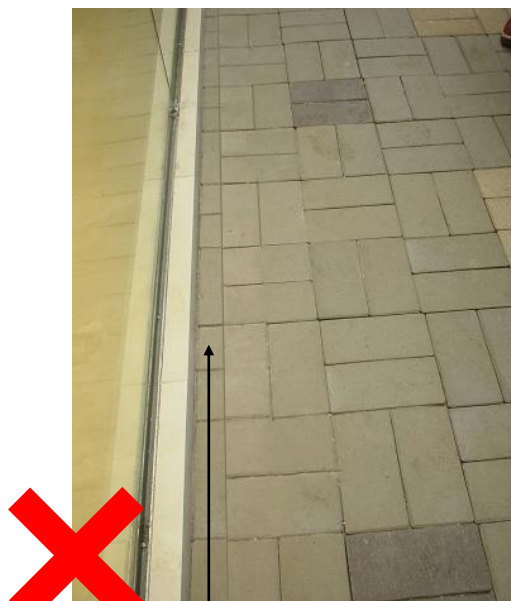
Poor practice for cut less than \frac{1}{3} of a block size
