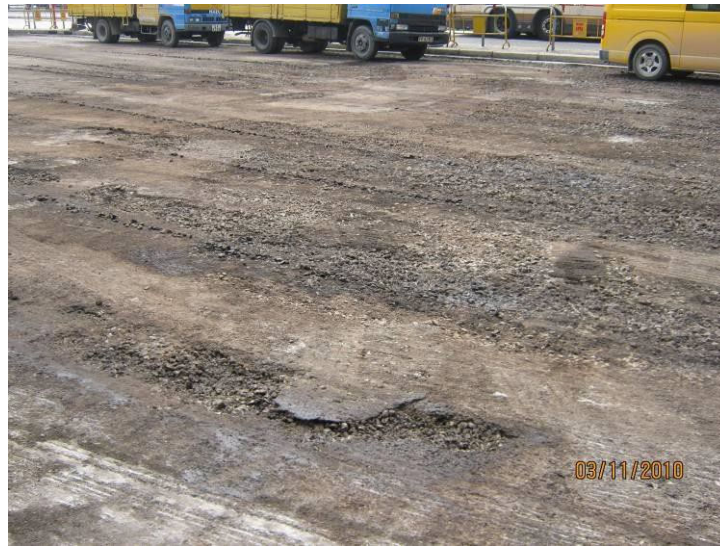
Photo 3 – Disintegrated base layer materials exposed after coldmilling
