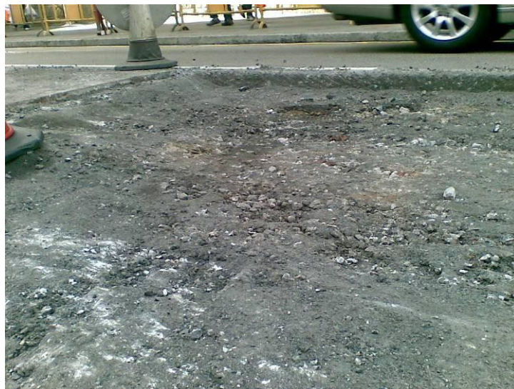
Photo 4 – Disintegrated base layer materials exposed after coldmilling
