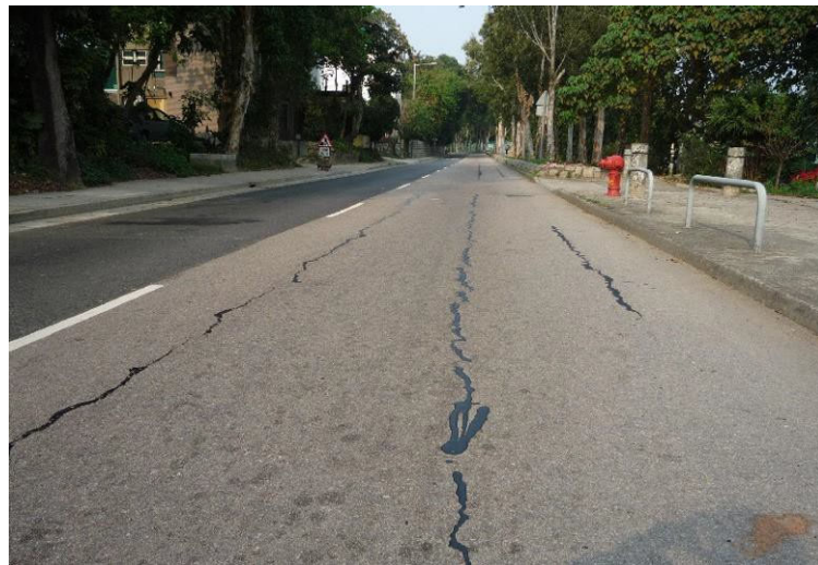
Photo 1 – Filling of wide single longitudinal cracks caused by the adjacent trench excavations
