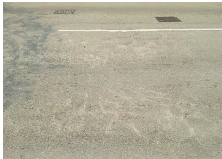
Photo 6 – Sign of pumping from lean concrete base
