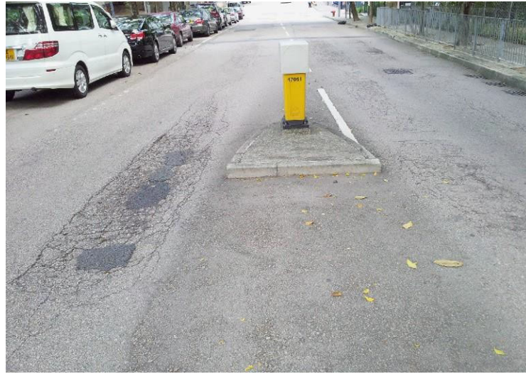
Photo 5 – Severe surface distress requiring deep inlay
