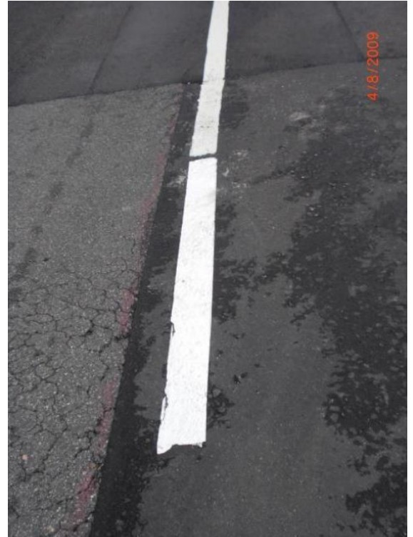
Plate 5: Road marking has not been properly reinstated.
