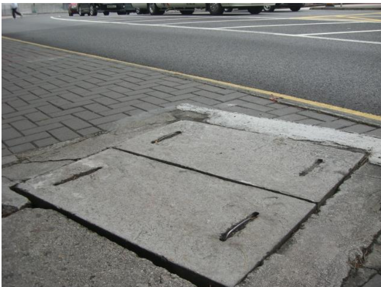
Plate 3: Block cracks were found on concrete slabs around drawpits.
