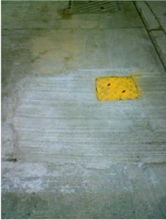
Plate 4: Saw cutting was not carried out.
