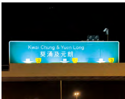
Gantry sign illuminated with LED lights
