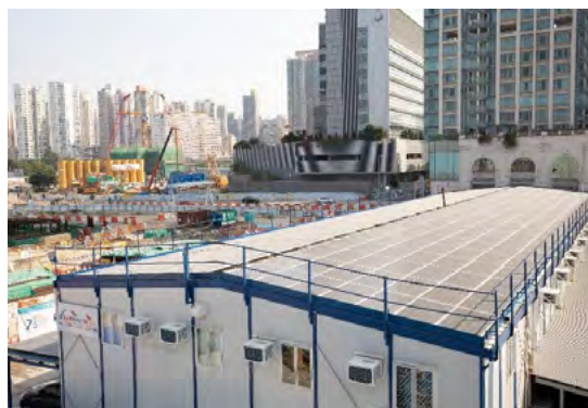
Solar panels on the roof of the site office and car park of Contract No. HY/2014/20
