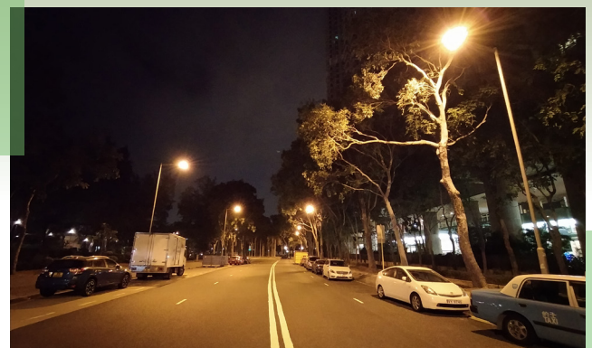
▲ Conventional High Pressure Sodium lights at Man Tung Road in Tung Chung
