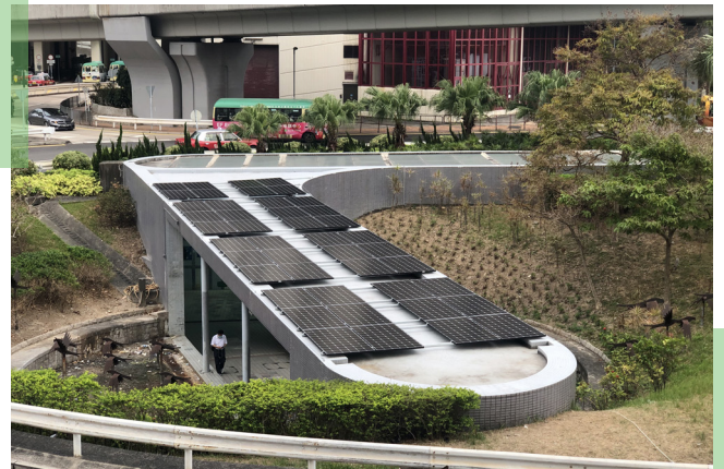
▲ PV system on an existing subway in Kwai Fong
