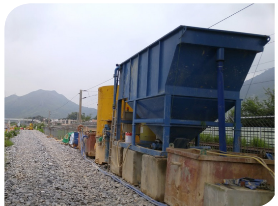
Deploy wastewater treatment facilities to treat wastewater before discharging
