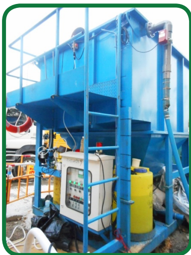
Wastewater Management - Wastewater treatment facilities on site
