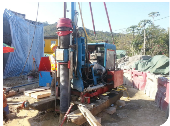
Noise enclosure to reduce noise impact
