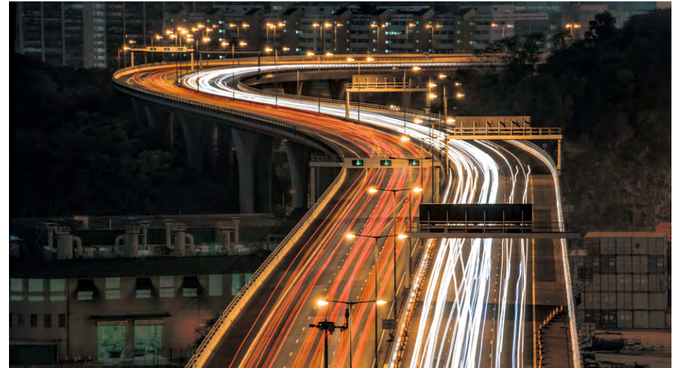
Public lighting for highways
