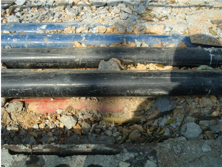
Photo 1 – PVC Duct (NWT)
