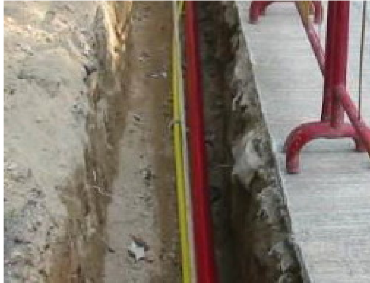
11kV & Pilot Cables
