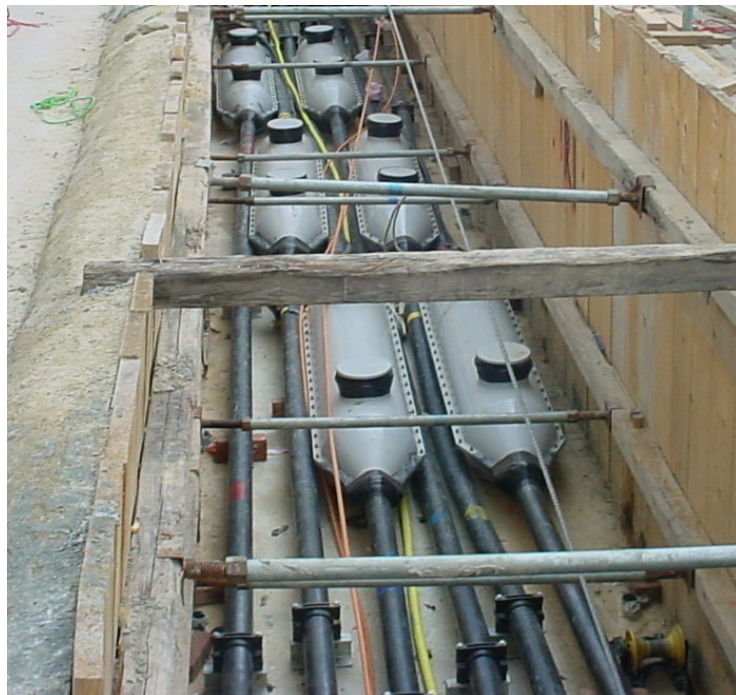
132kV Cable & Joint
