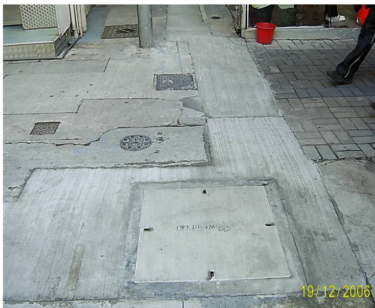
Photo No.1 (Joint Box - Concrete Type) Covers Number: from 1-3
