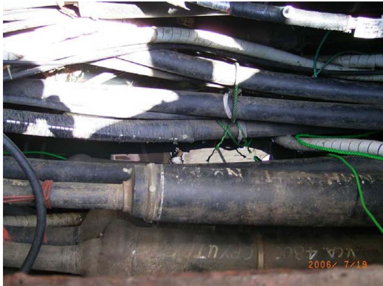
Photo No. 5 (Cables)
