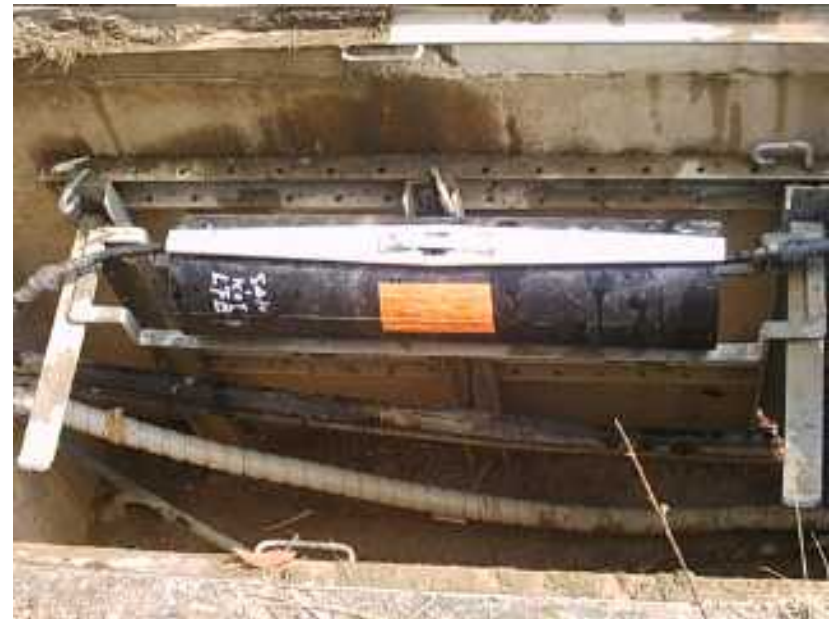
Photo No. 6 (Cable Joint)
