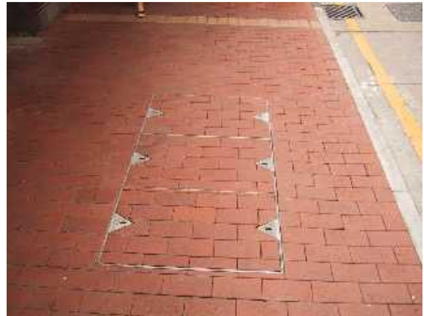
Photo No. 8 (Manhole/Joint Box – Recessed Type) Covers Number : from 1-5
