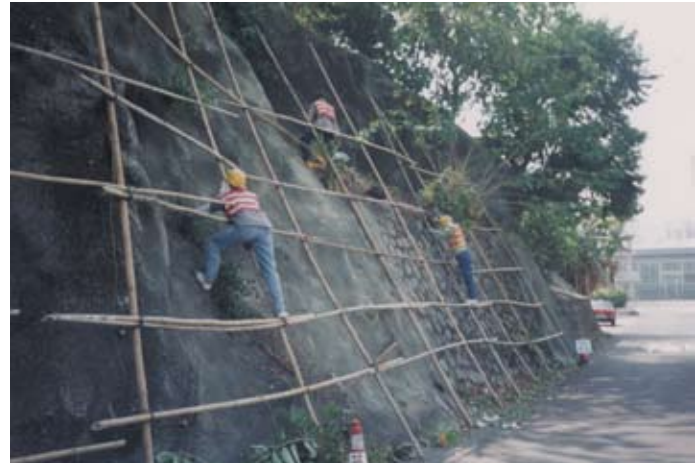
清理路旁斜坡上的排水孔及修補斜坡護面的裂痕 Cleaning blocked weepholes and repairing cracked surfacing on a roadside slope
