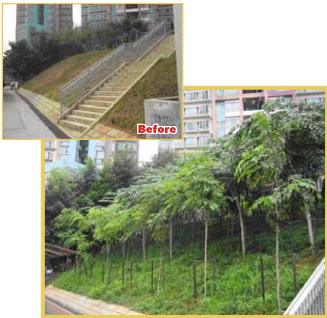
Improvement planting work on slope 6NW-C/C288 along Castle Peak Road - Langnan, Tuen Mun
