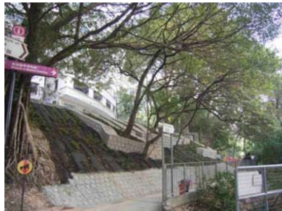
Slope No. 11SW-A/FR135 at Caine Lane – Preservation of existing trees in-situ as part of the slope upgrading works
