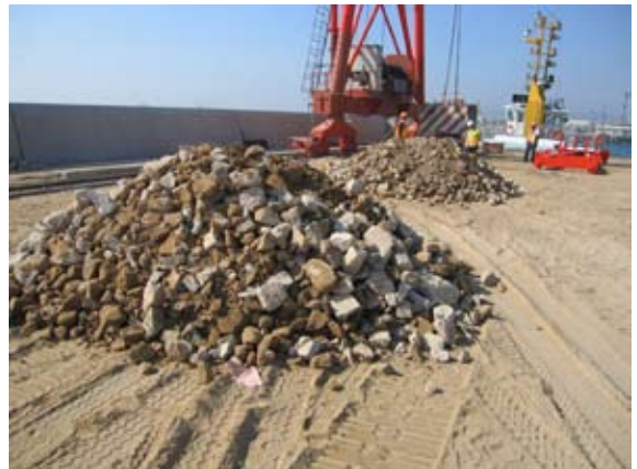
Using of recycled grade 200 rock fill from Public Filling Area as temporary road sub-base
