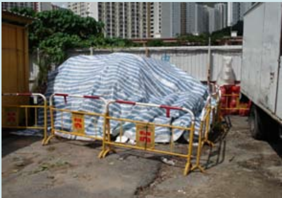
Dusty material covered up
